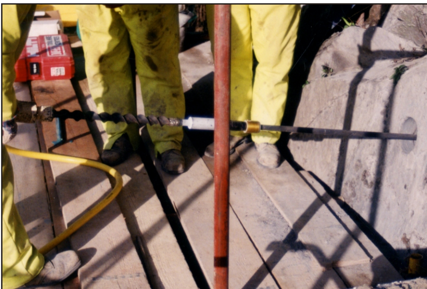
Fibregrip® Rockbolt being spun through the capsules to mix the resin. The remainder of the hole was post grouted 24 hours later.
